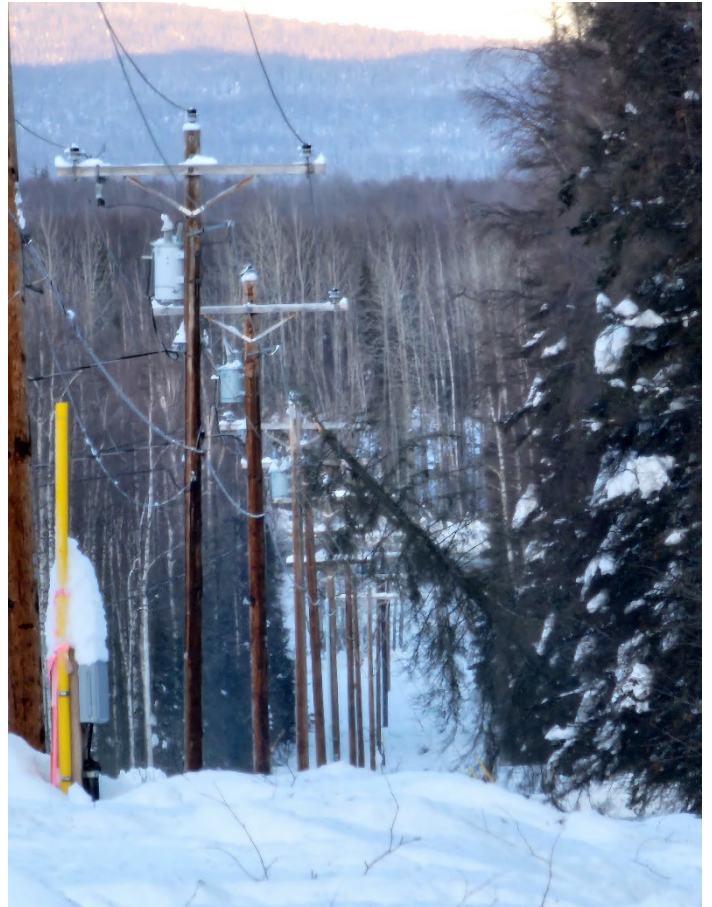
Wind-blown tree fallen into power lines on Dodge Dr
